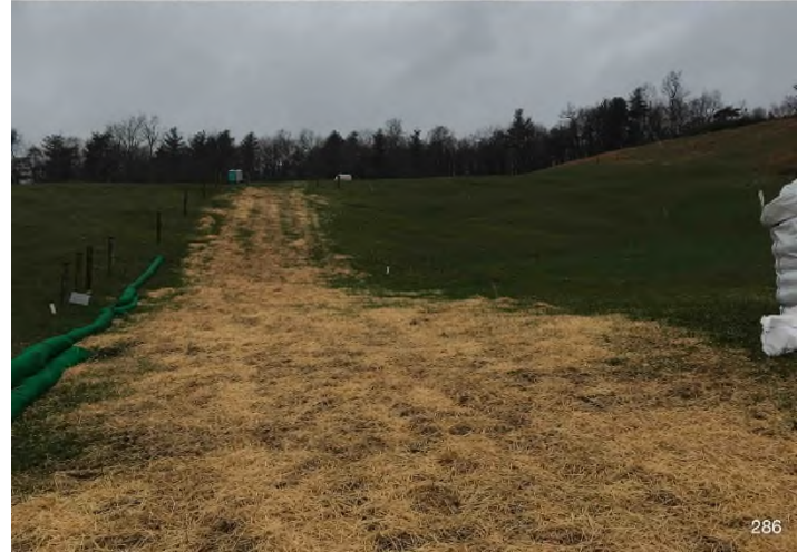
Figure 2: MVP-RO-286 – Controls in place and functioning properly. BRG: 275°W (T) LAT: 37.144866 LON: -80.135835 ±16ft ALT: 2684ft
