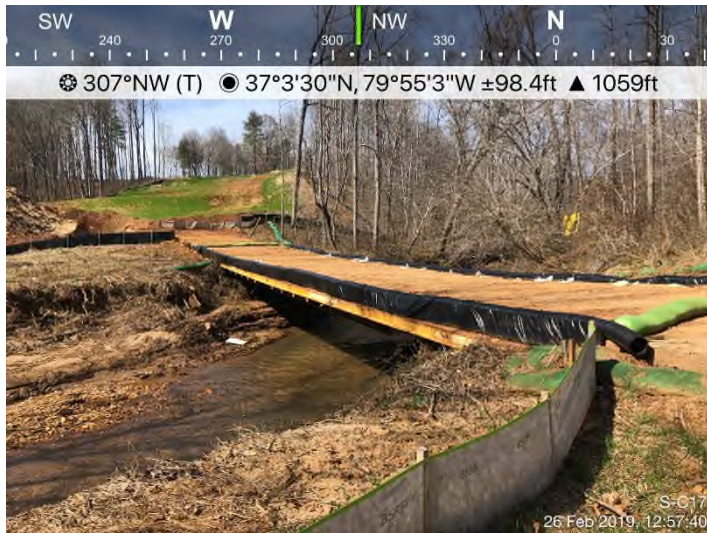
Fig. 9: S-C17 – Controls in place.
