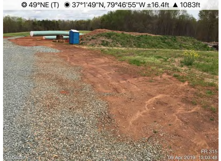
Fig. 10: STA 14411+04 – MVP-FR-315: Stabilize along shoulder.
