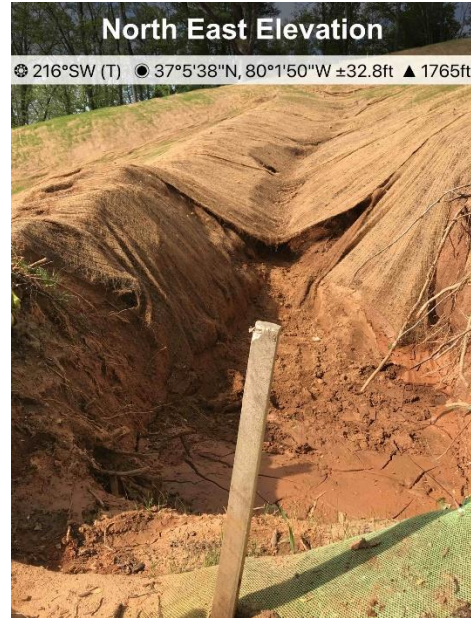
Fig. 2 St#13404+00 waterbar and sump requires maintenance
