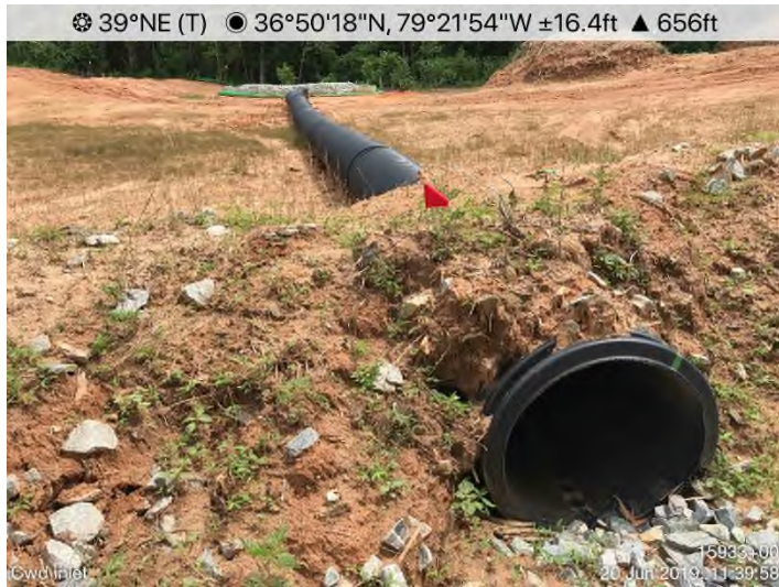
Fig. 9: STA 15933+00 – CWD inlet not functioning.
