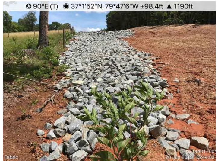
Fig. 10: STA 14401+00 – Riprap channel does not have fabric underlayment.
