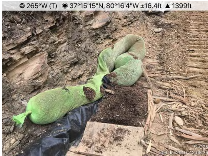
Fig. 5: STA 12163+05 – CFS “Waddles” need maintenance at stream S-C25.
