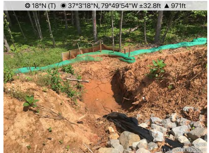
Fig. 6: STA 14229+00 – Sump maintenance needed.
