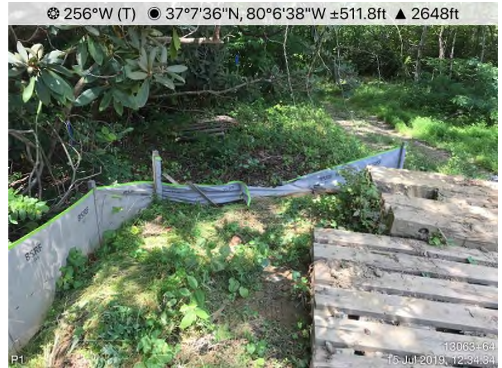
Fig. 10: STA 13063+64 – P1 in repair needed.
