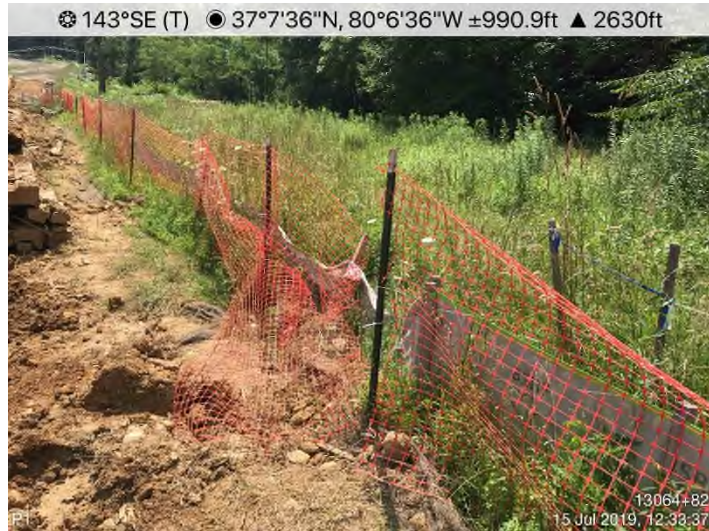
Fig. 9: STA 13064+82 – P1 in repair needed.
