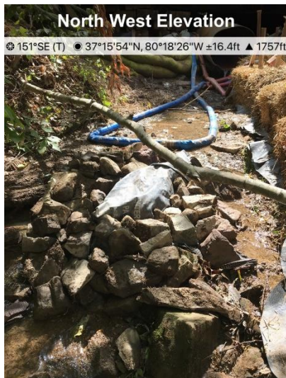
Fig. 3 Designated stream SG-40 pump around energy dissipater
