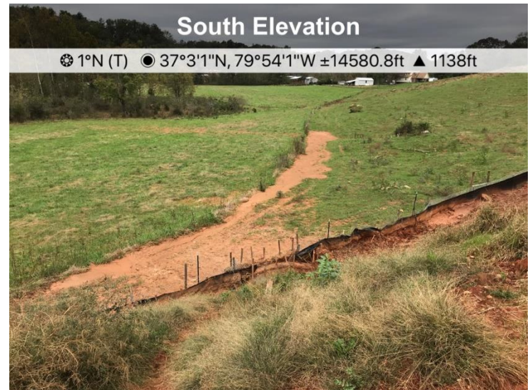
Fig. 2 At St#13903+00 sediment has left the ROW.
