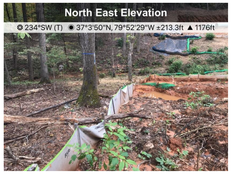
Fig. 4 At St#14067+96 the P1 requires maintenance.
