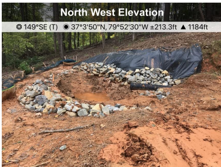
Fig. 3 At St#14065+80 sump is not installed per the redline sizing.
