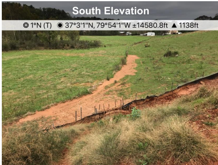
Fig. 9 At St#13903+00 sediment has left the ROW.
