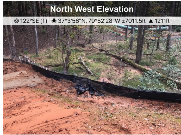
Fig. 2 At St#14064+80 sediment has left the ROW.
