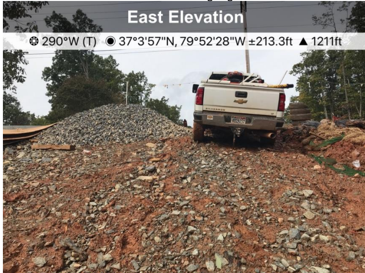
Fig. 1 The CE at St#139201+00 is showing signs of erosion.
