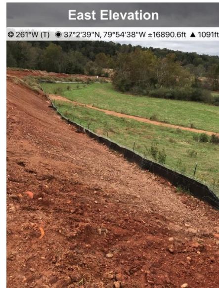
Fig. 10 The area between 13903 and St#13926 lacks stabilization.
