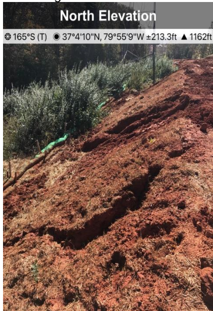
Fig. 3 At 13824+50 slope is not adequately stabilized and is eroding
