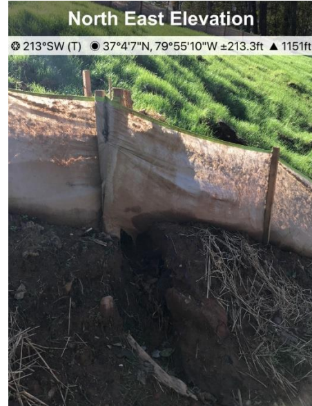
Fig. 2 At 13818+62, undermined silt fence
