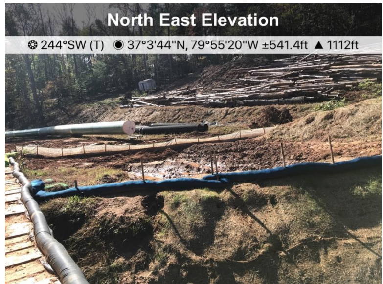
Fig. 4 At designated stream S-C14 stream buffers not adequately stabilized.
