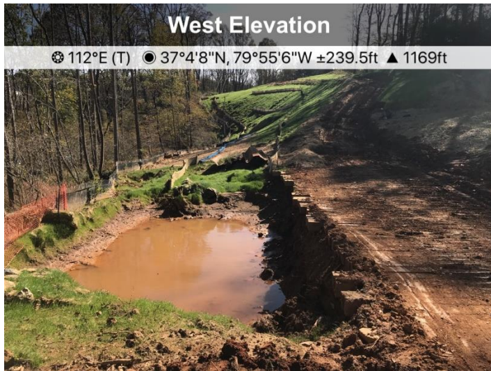
Fig. 1 At St#13817+00, sump is not completed
