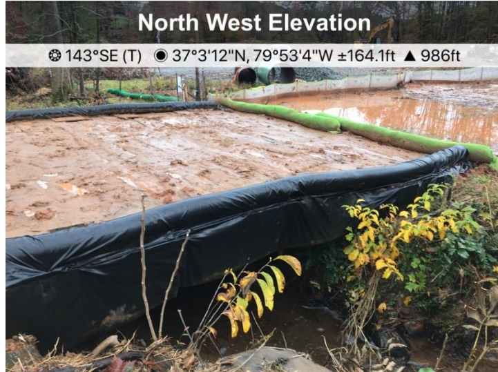
Fig. 1 Designated stream crossing SKL36, bridge liner is filled with sediment.
