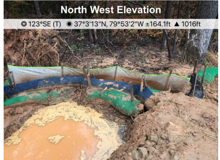
Fig. 2 At St#14001+04 ECD requires maintenance and sediment removal off ROW.
