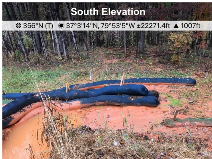
Fig. 3 At St# 14082+06 ECD requires maintenance and sediment removed off ROW.
