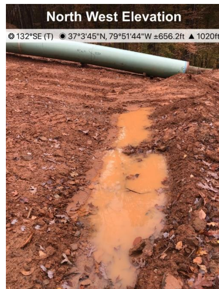
Fig. 4 At St# 14106+00 water bar requires maintenance and to be built back to spec.
