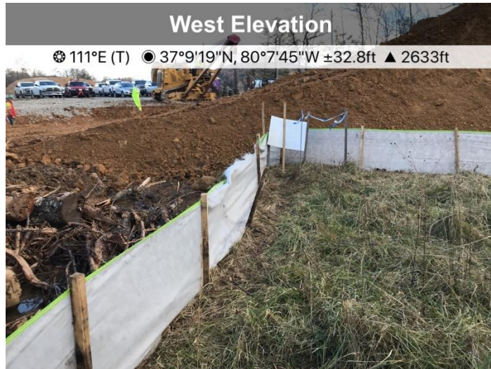
Fig. 1 Torn silt fence at St#12865+11
