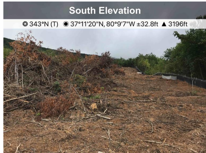
Fig. 2 St12712 lacks stabilization
