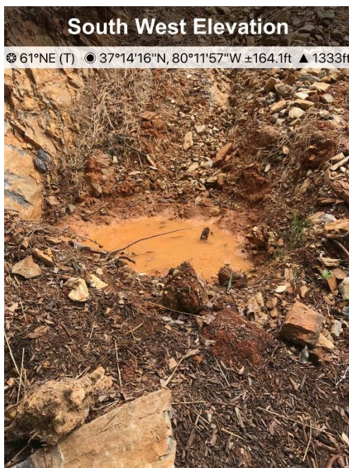
Fig. 3 St12417+00 sump lacks adequate capacity
