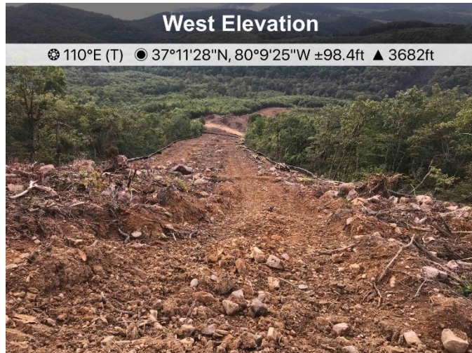
Fig. 1 St12690 lacks stabilization
