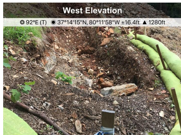
Fig. 4 St12418+00 sump lacks adequate capacity
