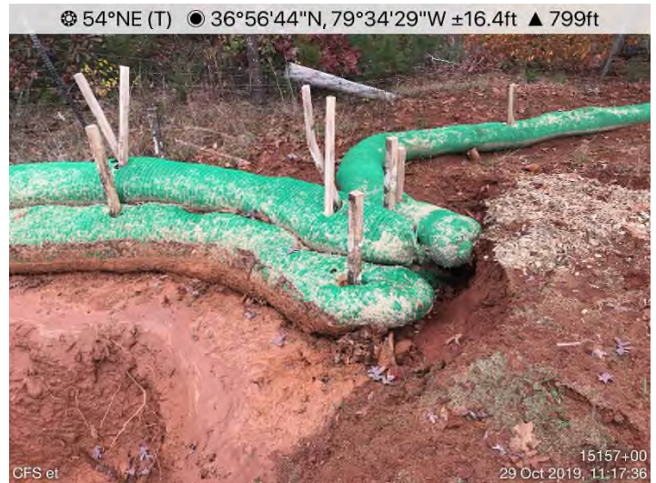
Fig. 10: STA 15157+00 – CFS end-treatment bypassed. Maintenance needed.
