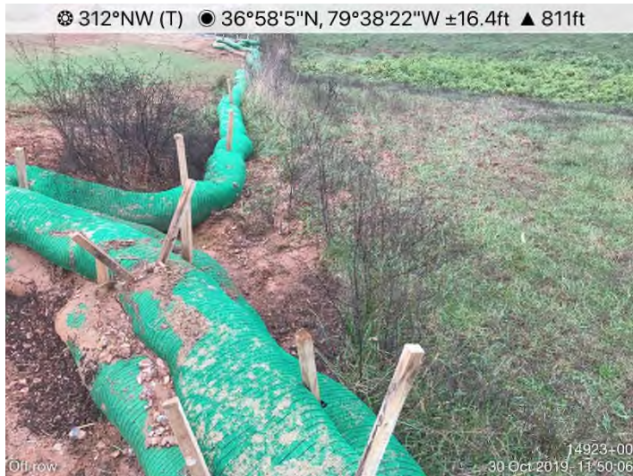
Fig. 25: STA 14923+00 – Sediment off ROW.
