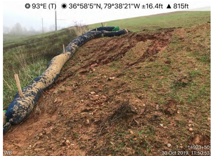
Fig. 26: STA 14923+50 – Waterbar maintenance needed.
