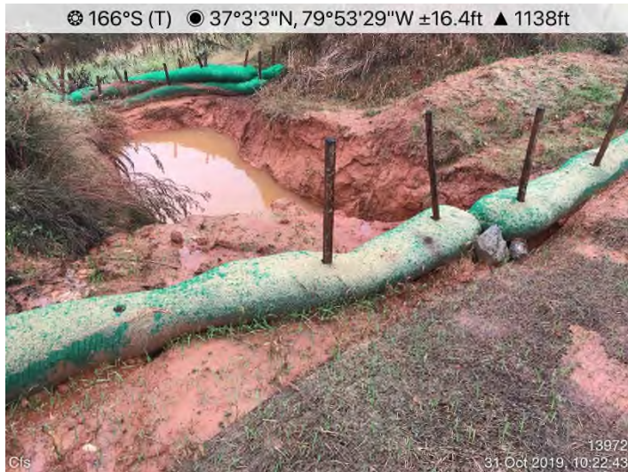
Fig. 5: STA 13972+00 – CFS maintenance needed.
