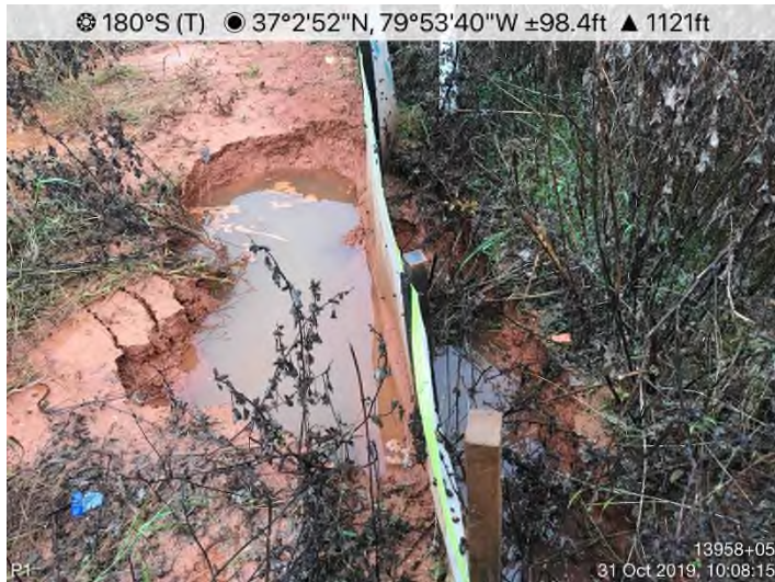
Fig. 1: STA 13958+01 – P1 maintenance needed.
