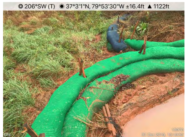
Fig. 4: STA 13970+00 – CFS maintenance needed.
