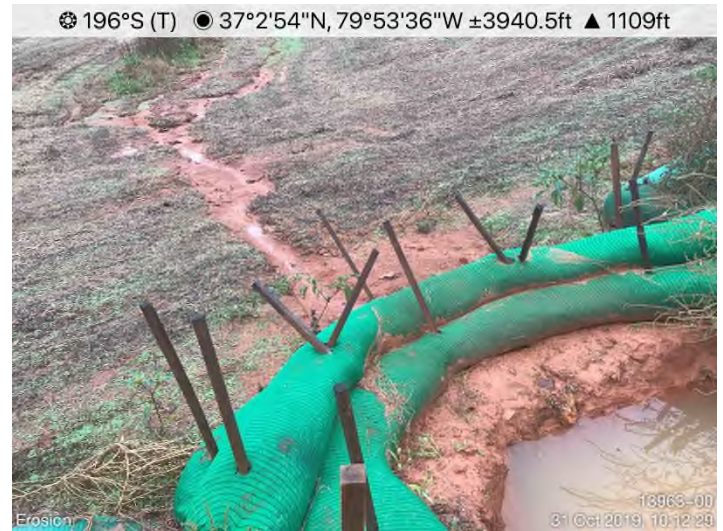
Fig. 2: STA 13963+00 – End treatment causing scour outside of LOD.
