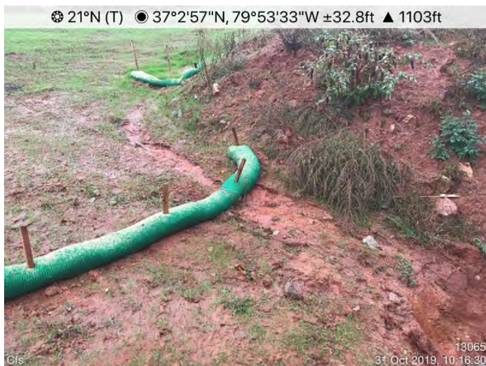
Fig. 3: STA 13965+00 – CFS maintenance needed.
