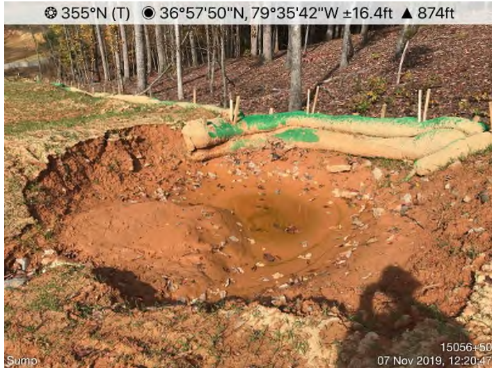
Fig. 5: STA 15056+00 – Sump maintenance needed.
