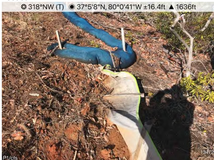
Fig. 3: STA 13472+00 – P1 and CFS maintenance needed.
