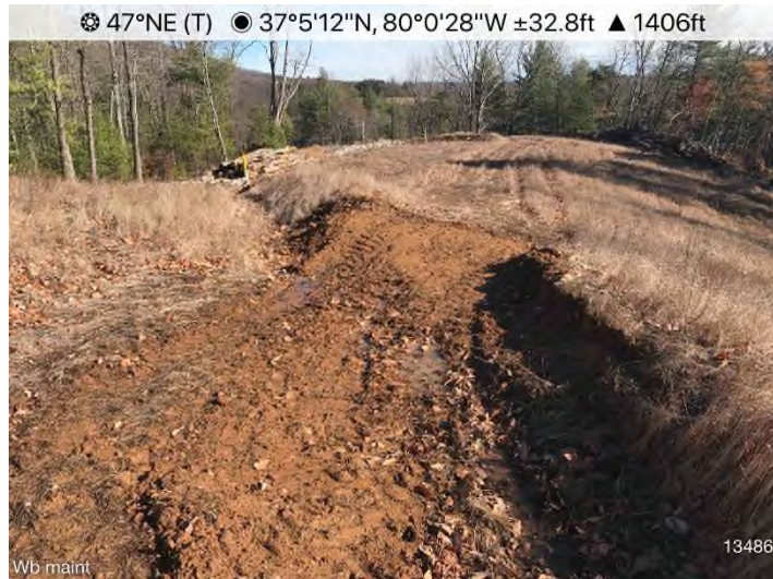
Fig. 5: STA 13486+00 – Waterbar maintenance needed.
