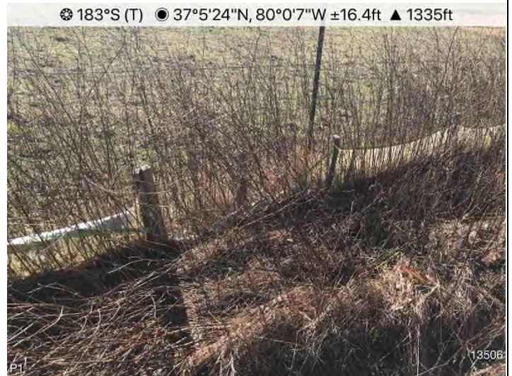
Fig. 6: STA 13506+00 – P1 maintenance needed.
