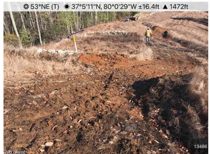
Fig. 4: STA 13485+50 – Waterbar maintenance needed.
