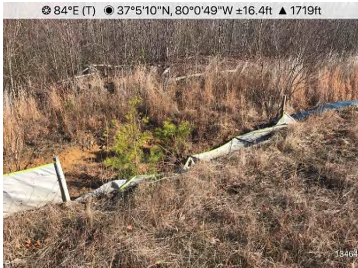
Fig. 1: STA 13464+00 – P1 maintenance needed.
