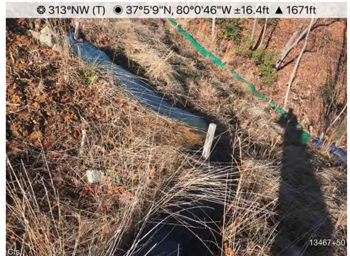
Fig. 2: STA 13467+50 – CFS maintenance needed.
