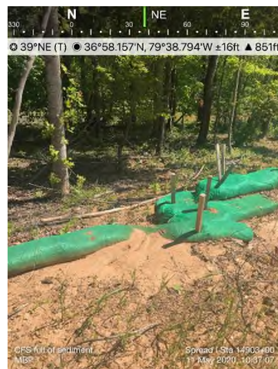
Figure 6: STA 14903+00 – CFS at capacity.
