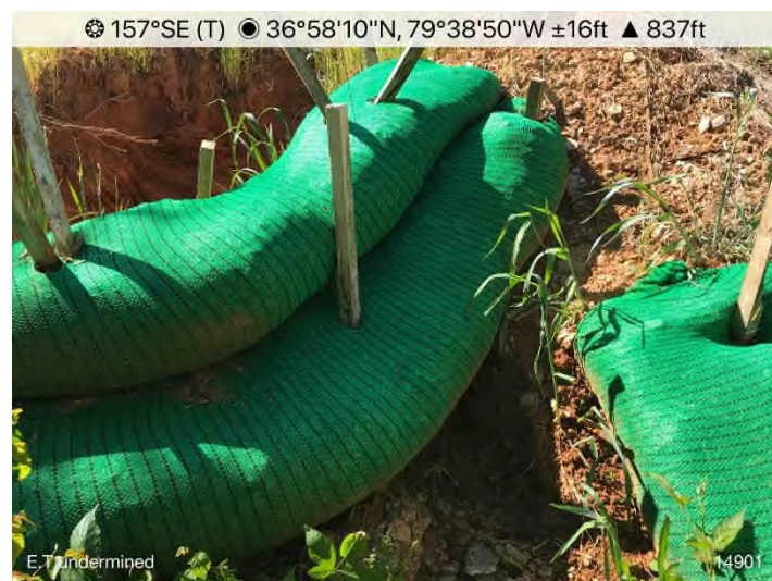
Figure 5: STA 14901+00 – End-treatment undermined.
