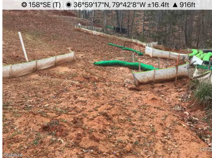
Figure 1: STA 14717+50 – Re-stabilize denuded ROW and repair erosion.
