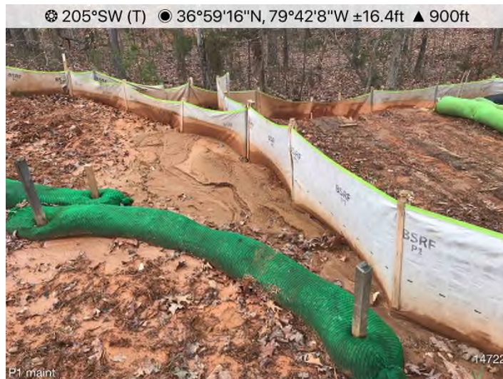
Figure 3: STA 14717+50 – P1 maintenance needed.
