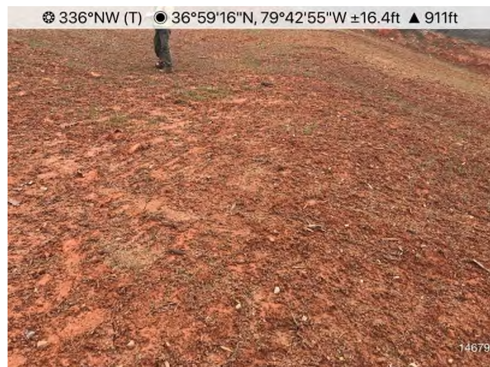
Figure 5: STA 14679+00 – Waterbar maintenance needed.
