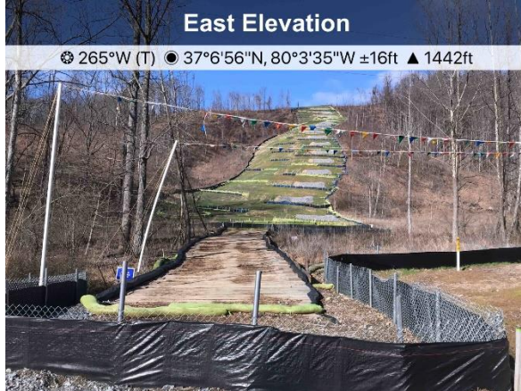
Figure 1: Designated crossing S-II4, ECD's are in place.
