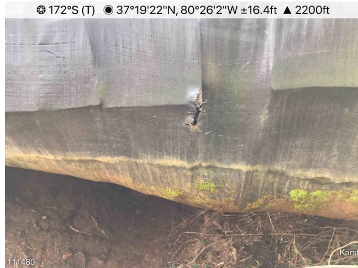
Figure 17: STA 11480+00 – Bridge underlayment repair needed.
