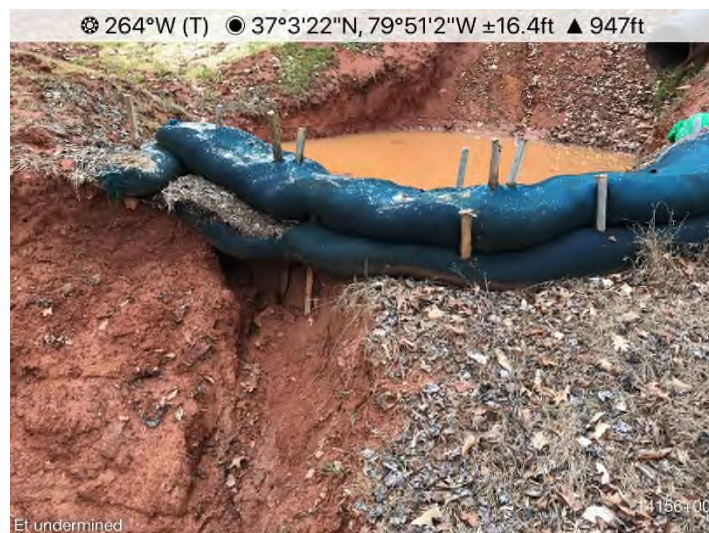
Figure 14: STA 14156+00 – End Treatment undermined. Maintenance needed.
