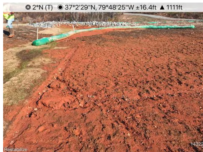
Figure 6: STA 14322+00 – Re-stabilization needed.
