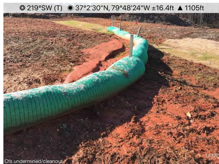
Figure 5: STA 14322+00 – CFS undermined. Repair needed.
