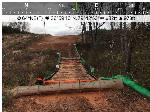
Figure 4: Designated crossing S-H37, ECD's are in place.
