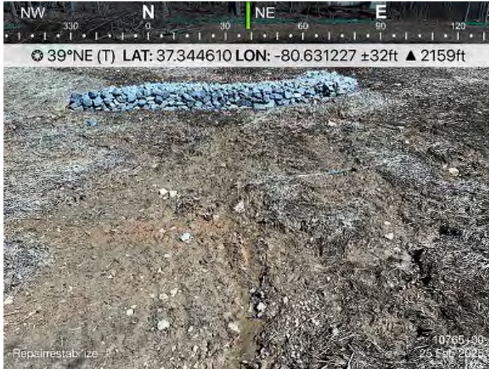
Fig. 1 STA 10765+00: Restabilize and repair rill erosion.
