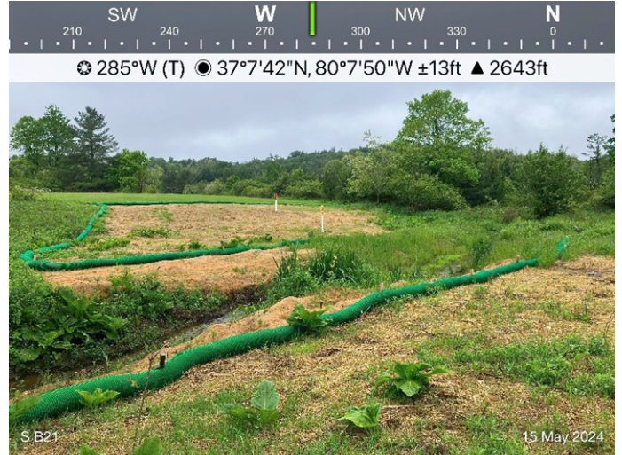
Figure 4: Designated crossing S-B21, ESC's devices in place.
