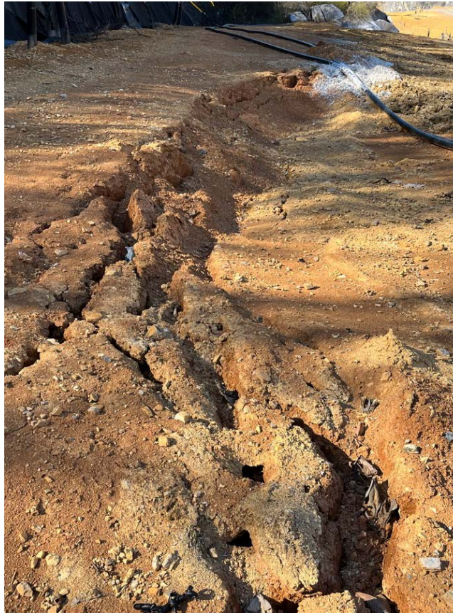
Figure 10 - Scarp and Settlement Cracks
