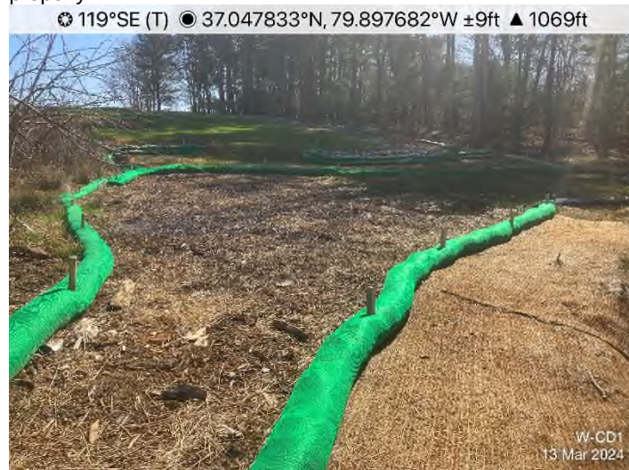
Figure 3: Wetland W-CD1 – Controls in place and functioning properly.
