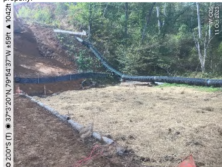
Figure 3: Wetland W-CD5 – Controls in place and functioning properly.
