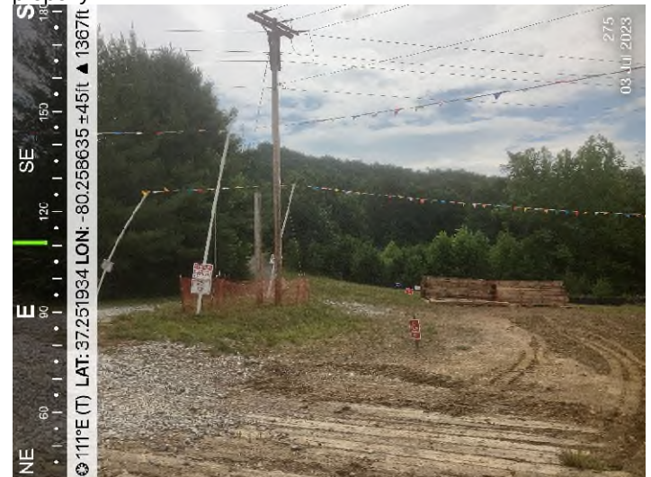
Figure 4: MVP-MN-275 – Controls in place and functioning properly.
