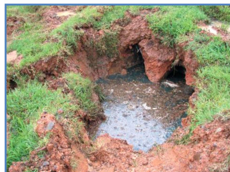
Failed Septic System
