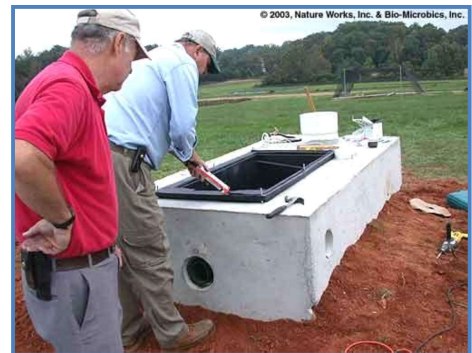
On-site Sewage Disposal System
