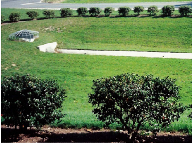
Figure 7. Extended detention basin (Photo: USEPA)
