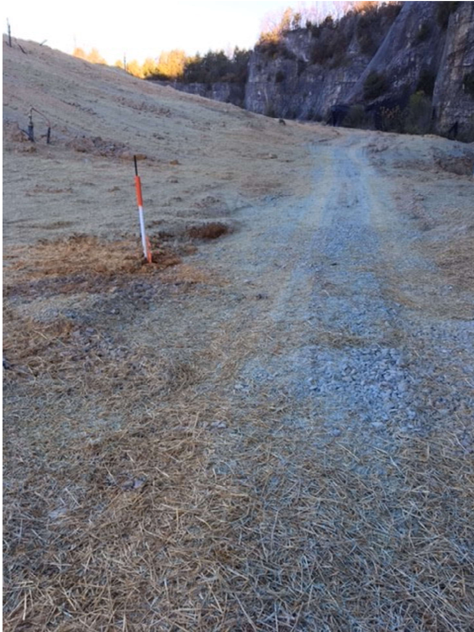
Settlement plate installed near leachate collection tank (LCT-1).
