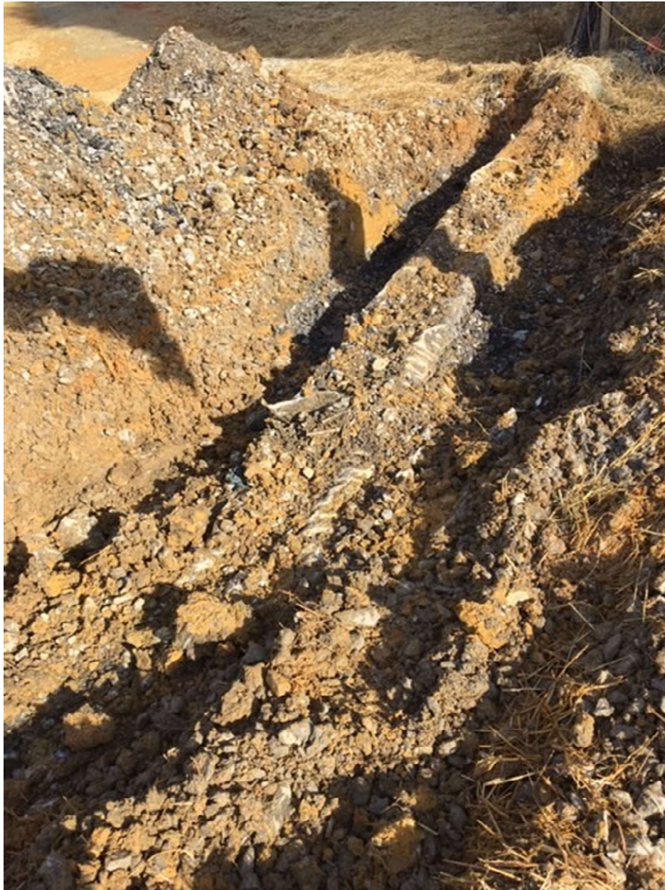
LFG header (8-inch) road crossing to wells GW-36 and GW-65. Header regraded and vacuum reestablished to wells.
