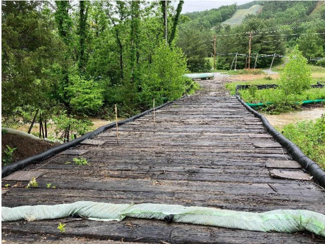
Figure 1: Designated crossing S-C21, ECD's are in place.
