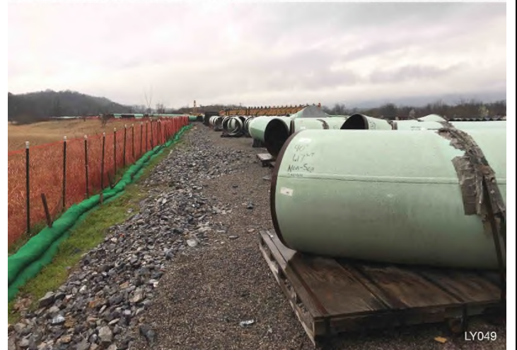
Figure 4: Laydown Yard 049 – Controls in place and functioning properly. BRG: 279°W (T) LAT: 37.275588 LON: -80.113424 ±7450ft ALT: 1201ft
