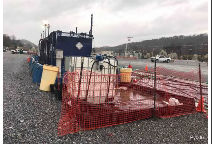
Figure 2: Pipe Yard 006 – Controls in place and functioning properly. BRG: 292°W (T) LAT: 37.235592 LON: -80.226649 ±32ft ALT: 1254ft
