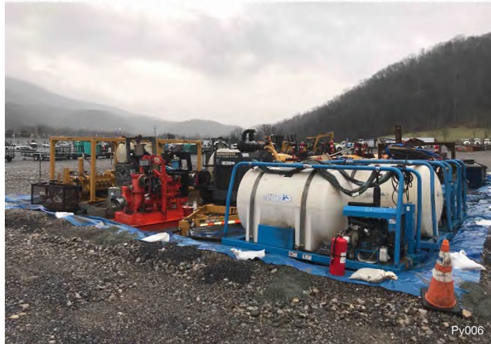
Figure 3: Pipe Yard 006 – Controls in place and functioning properly. BRG: 51°NE (T) LAT: 37.234104 LON: -80.228112 ±164ft ALT: 1290ft
