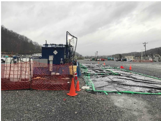
Figure 1: Laydown Yard 06, fueling area is protected.
