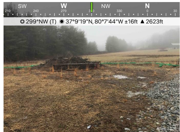
Figure 4: ATWS 1326, ECD's are in place and functioning.
