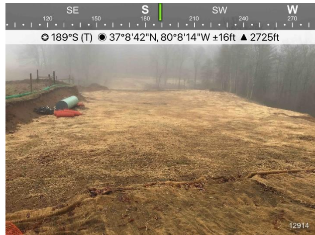
Figure 2: St12914, ESC controls were in place.
