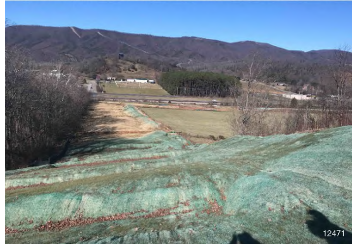
Figure 4: STA 12471+00 – Controls in place and functioning properly. Area stabilized with erosion matting. BRG: 353°N (T) LAT: 37.227036 LON: -80.202321 ±32ft ALT: 1322ft
