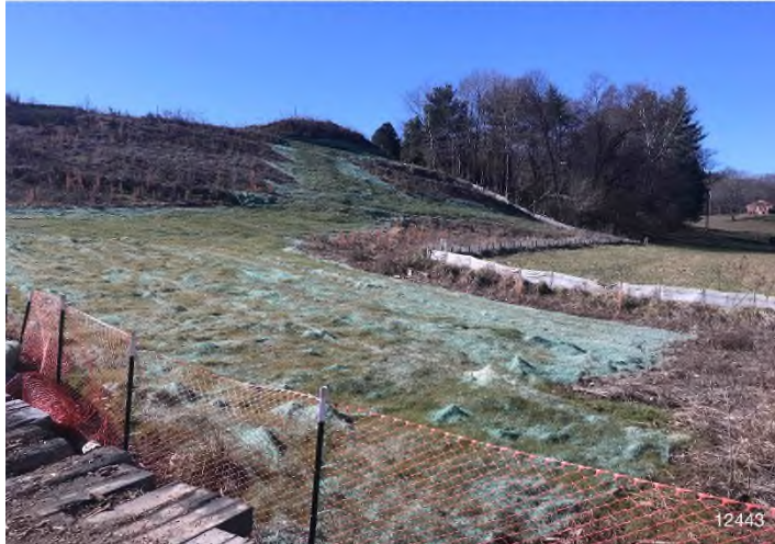
Figure 3: STA 12443+00 – Controls in place and functioning properly. Area stabilized with erosion matting. BRG: 295°NW (T) LAT: 37.233211 LON: -80.198265 ±958ft ALT: 1161ft
