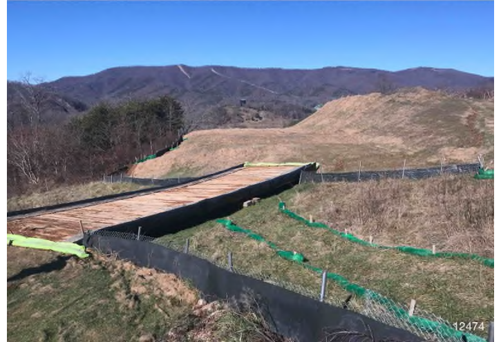
Figure 2: STA 12474+00 – Controls in place and functioning properly. Area stabilized with erosion matting. BRG: 334°NW (T) LAT: 37.226016 LON: -80.202059 ±32ft ALT: 1380ft
