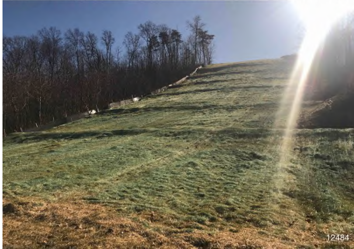
Figure 1: STA 12484+00 – Controls in place and functioning properly. Area stabilized with erosion matting. BRG: 136°SE (T) LAT: 37.223450 LON: -80.202113 ±16ft ALT: 1483ft
