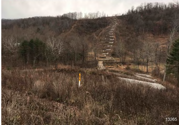
Figure 1: STA 13265+00 – Controls in place and functioning properly. BRG: 86°E (T) LAT: 36.990646 LON: -80.064500 ±23727ft ALT: 1413ft
