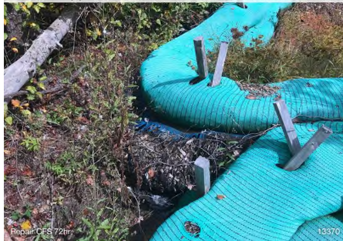
Figure 4: STA 13360+00 – CFS maintenance needed. BRG: 41°NE (T) LAT: 37.101490 LON: -80.036315 ±16ft ALT: 1706ft
