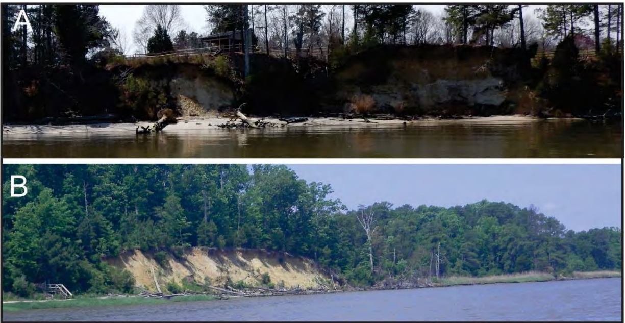
Figure 4-4. A) Eroding banks at the Visitor's Center along Reach 2. B) Reach 2 is a mix of intermittent eroding uplands and marsh shorelines.
